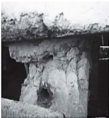
Figure 3. Destruction of foundation pile structures as a result of swamping (Yakutsk, 2008) [4, p.29].
