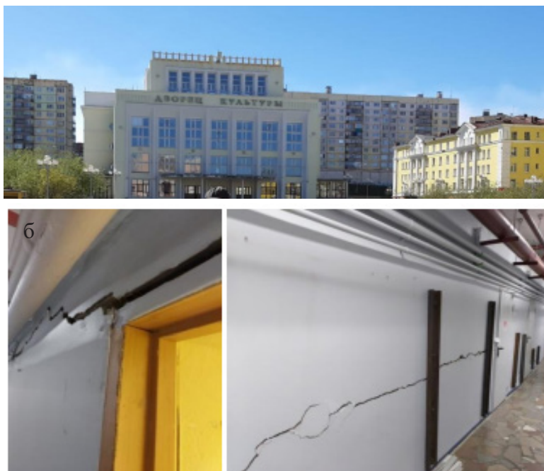
Figure 1. The facade of the building of the Palace of Culture in Norilsk (a) and the resulting cracks in the building (b) (data as of summer 2021) [1, p. 27].
