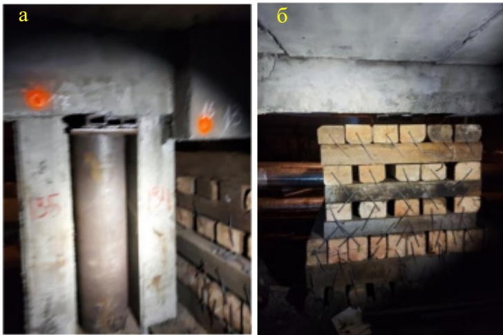
Figure 2. The basement of the building of the Palace of Culture [1, p.28]: a - additional supports; b - cages from sleepers
